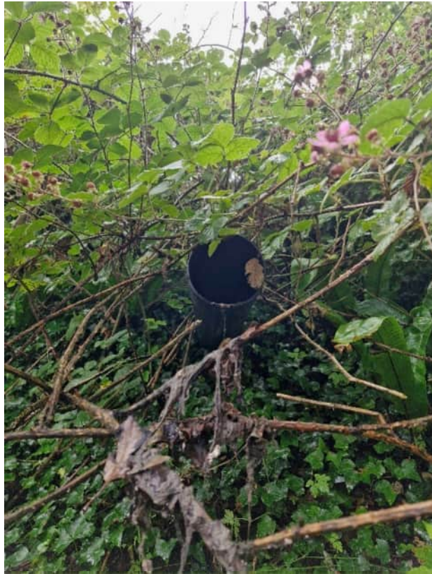
Plate 4 Pipe outflow at SW1 sampling location
